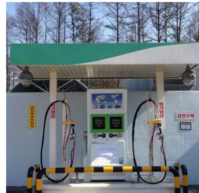
Fueling station (capacity : 250Nm 3 /h)
