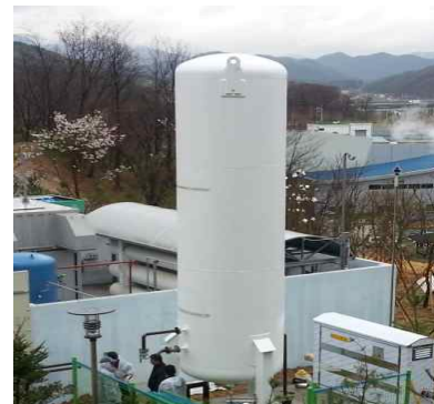
Buffer Tank (15m 3 , 4~5bar)
