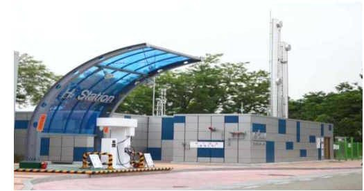
Sangam LFG-to-Hydrogen Station
