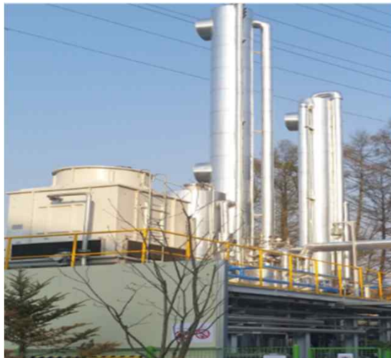
Biogas production facility (capacity : 600Nm 3 /h)
