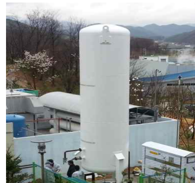
Buffer Tank (15m 3 , 4~5bar)
