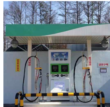
Fueling station (capacity : 250Nm 3 /h)
